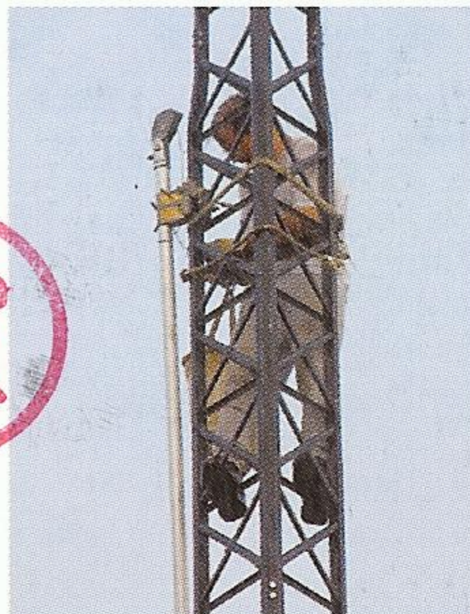
I usually just ride-out the frequent downpours on the tower. If you can't work in the rain in Barbados, you can't get anything done!
